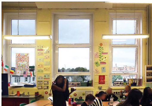
Poor: no external or internal shading control (left)
